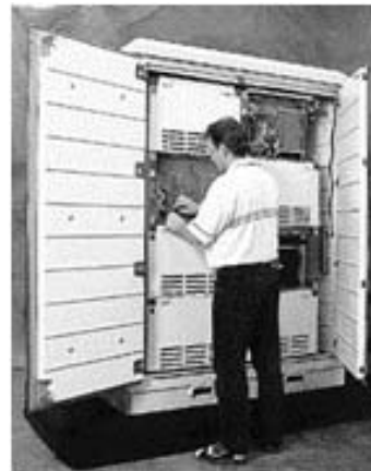
Dual band IS-136 Ericsson RBS 884 base station
